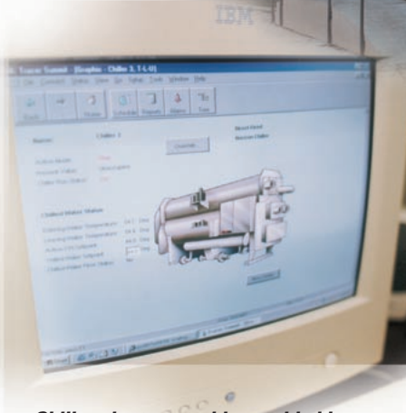
Chiller plant control is provided by a Tracer Summit system.
