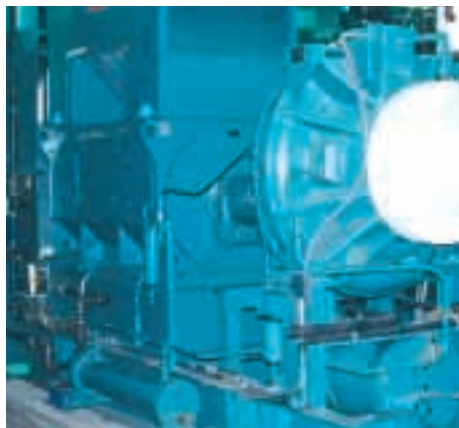
The 0.60 kW/TR efficiency rating of the new 2100-TR electric-drive chiller (left) from YORK significantly improves upon the 0.76 kW/TR rating of the original electric-drive chiller.
