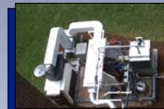
Combined heat and power systems providing electric or shaft power and thermal heat recovery
