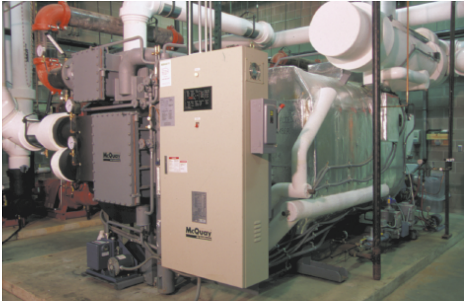
Oakview Middle School's 320-ton McQuay/Sanyo direct-fired natural gas absorption chiller
